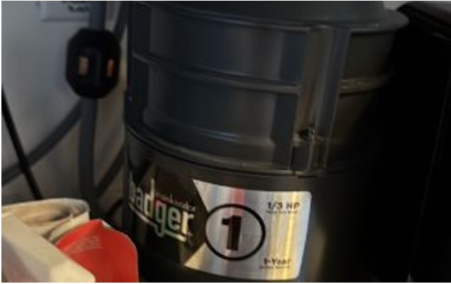
Under-sink garbage disposal (Badger 1/3 HP)
