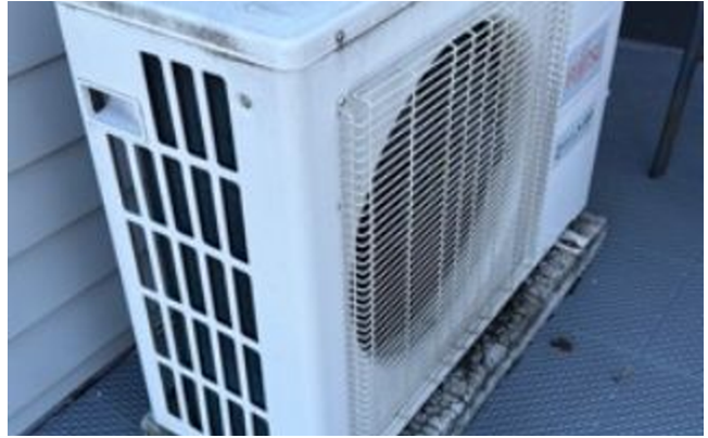
Outdoor Fujitsu condenser mounted on elevated pad
