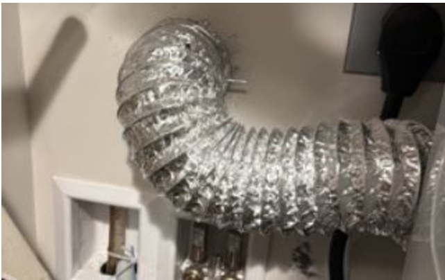
Laundry area vent duct and water connections.
