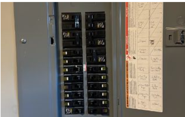
Main electrical service panel open
