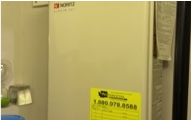
Water heater front view
