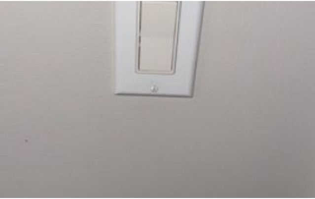
Loose switch plate
