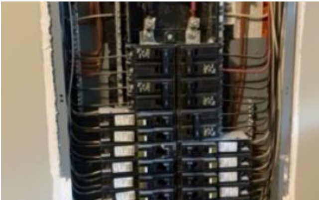
Main electrical service panel with cover removed
