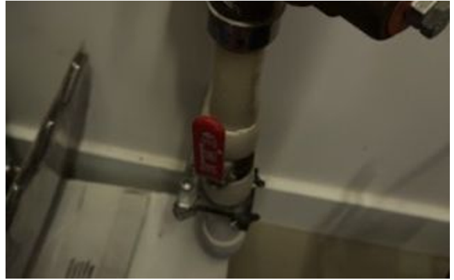
Cold water shutoff valve for water heater
